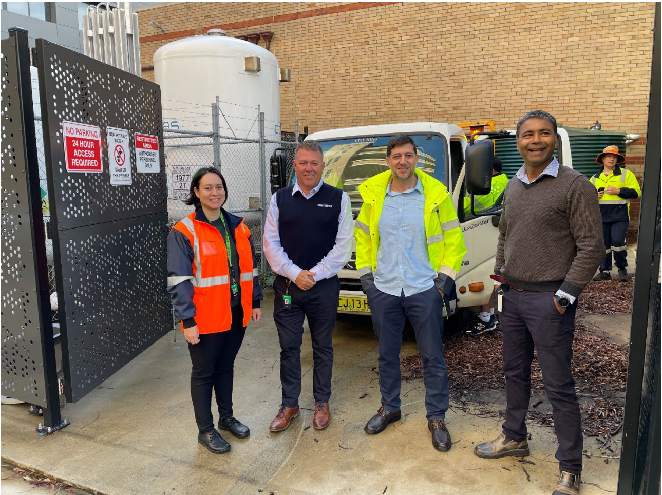
Royal Prince Alfred Hospital dialysis unit reverse osmosis water reuse fill point (Photo by Nicole Webb / City of Sydney)
